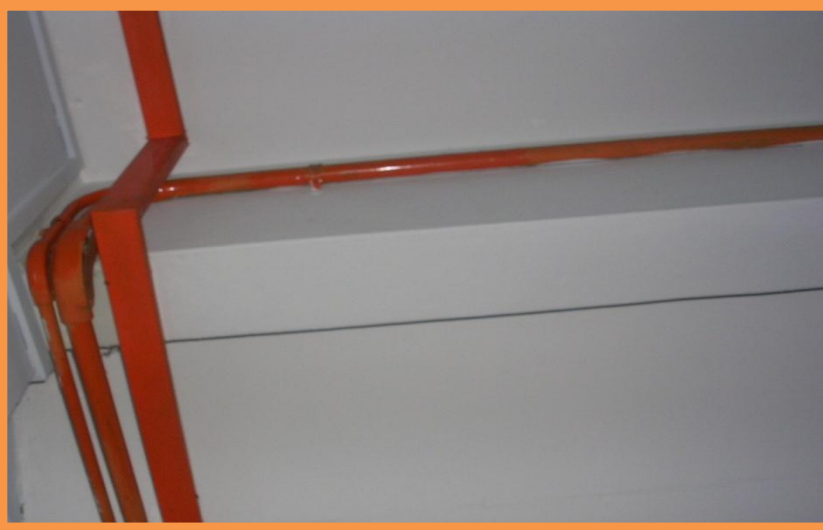
Run at ceiling level
